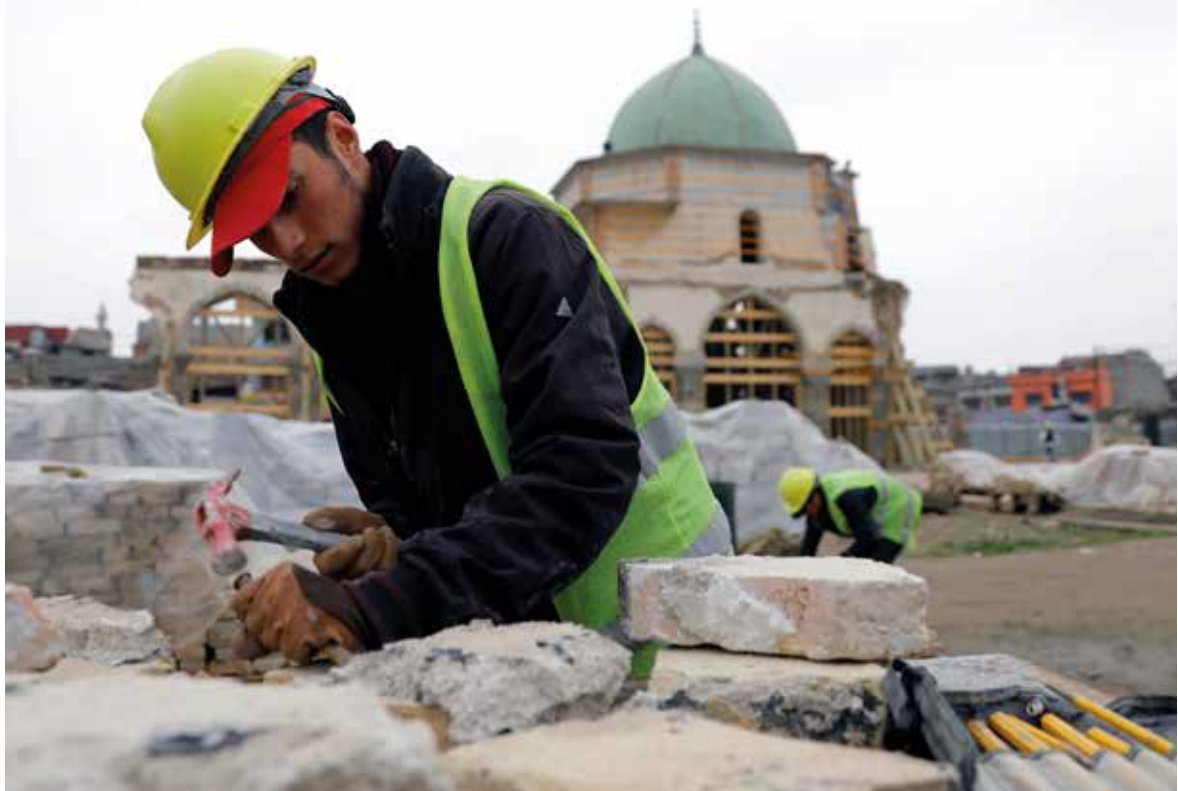
Reconstructing the Grand al-Nuri Mosque in the old city of Mosul, Iraq. Photo credit: Reuters
