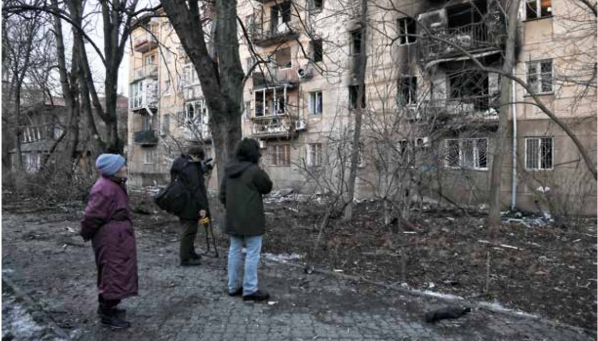
A residential building in Odessa damaged by a Russian drone attack, January 17, 2024. Photo credit: Nina Liashonok via Reuters Connect
